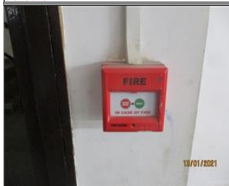
External photo(s) of the production unit(s) FIRE CALL POINT.JPG
