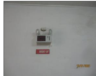
External photo(s) of the production unit(s) EMERGENCY LIGHT IN DINING HALL.JPG
