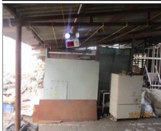
External photo(s) of the production unit(s) EMERGENCY LIGHTS NEAR BOILER WITH EXIT SIGNS.JPG
