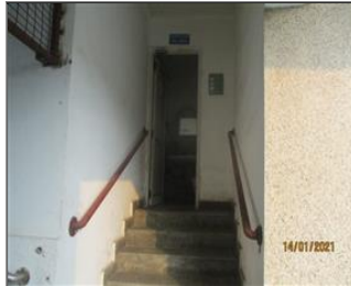
External photo(s) of the production unit(s) HAND RAIL PROVIDED TO TOILET STAIRS.JPG
