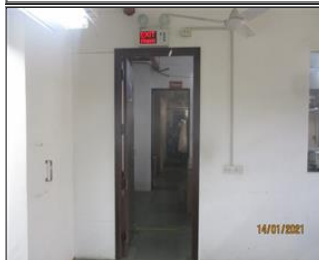
External photo(s) of the production unit(s) OUTWARD OPENING EXIT IN SAMPLING SECTION.JPG
