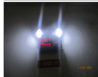
External photo(s) of the production unit(s) FUNCTIONAL EMERGENCY LIGHT IN DINING HALL.JPG
