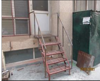
External photo(s) of the production unit(s) HAND RAIL PROVIDED TO STAIR CASE NEAR EMBROIDERY SECTION.JPG
