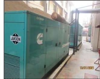
External photo(s) of the production unit(s) DIESEL GENERATOR.JPG
