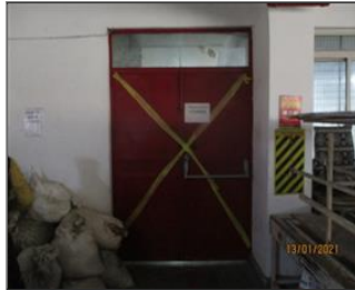
External photo(s) of the production unit(s) EMERGENCY EXIT ABANDONED FOR USE-EARLIER OPRNING IN DINING HALL.JPG
