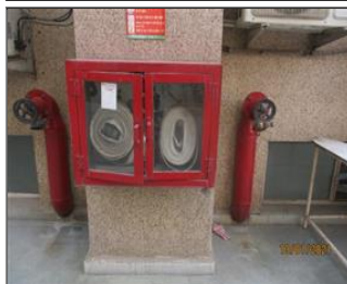
External photo(s) of the production unit(s) FIRE HYDRANT.JPG
